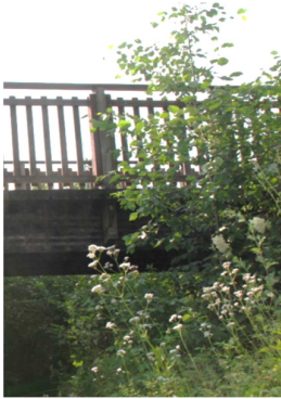
Figure 5.1. Bad detail, too much vegetation.
