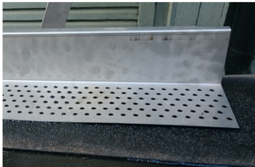
Figure 4.19. Steel angle with perforations in horizontal leg
