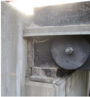
Figure 5.7. Bad detail, sill beam protrudes outside deck.
