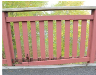
Figure 6.7. Rot in lower part of railing
