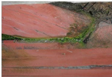
Figure 6.6. Growth of moss at connection
