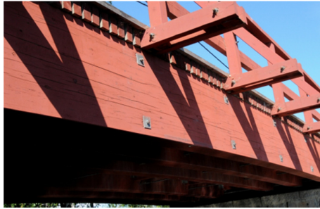
Figure 6.4. Painted glulam beam with some cracks
