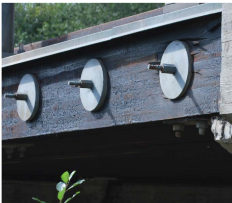
Figure 4.16. Creosote impregnated deck edge
