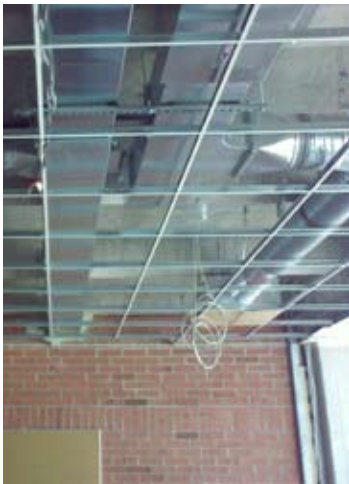
198. New ventilation system in the suspended ceiling
